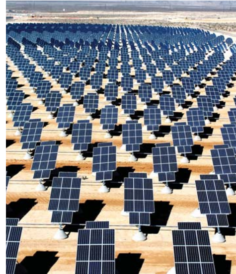
PV Field Array:
